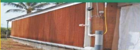
Evaporative Cooling System
