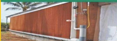
Evaporative Cooling System
