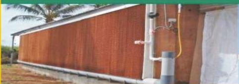
Evaporative Cooling System
