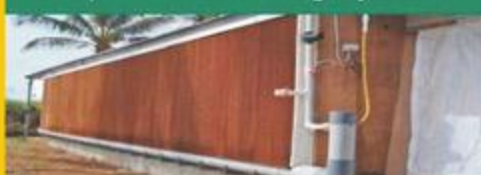
Evaporative Cooling System
