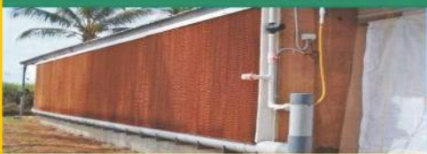
Evaporative Cooling System
