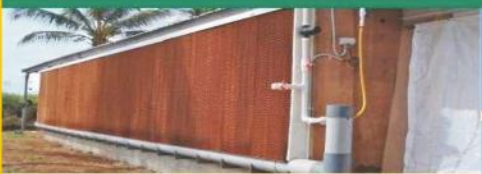
Evaporative Cooling System
